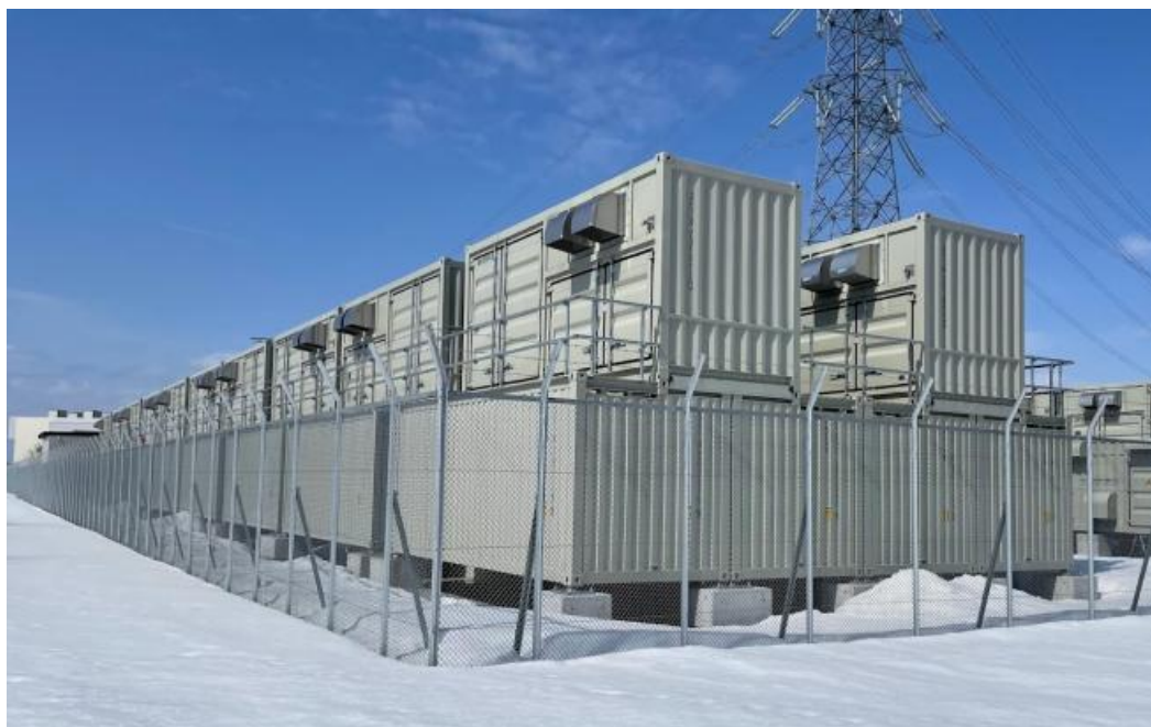
Figure 9: Sumitomo Electric Vanadium Redox Flow Battery 51 MWh plant in Hokkaido, Japan
