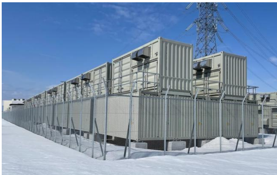
Figure 3: Sumitomo Electric Vanadium Redox Flow Battery 51 MWh plant in Hokkaido, Japan
